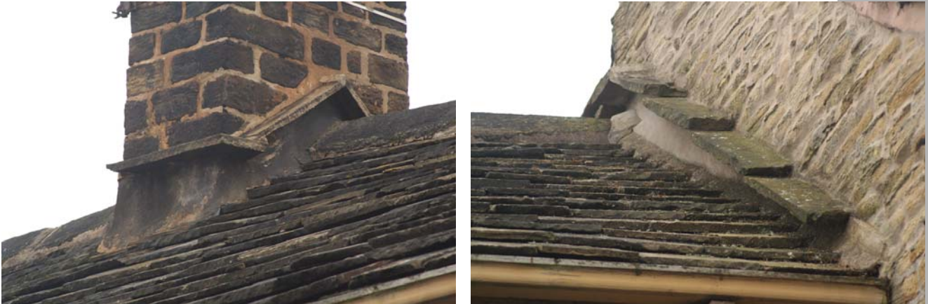
Water-tabling to gritstone chimneys (left) and thickstones to abutments (right) - local details
