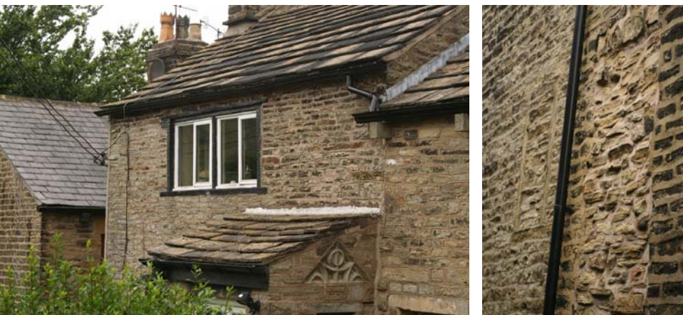
The former Seven Stars with four-light mullioned windows at first floor, extended eaves and additional headroom, and taking-in door in the gable (right) was probably in use as a domestic loomshop for weaving
