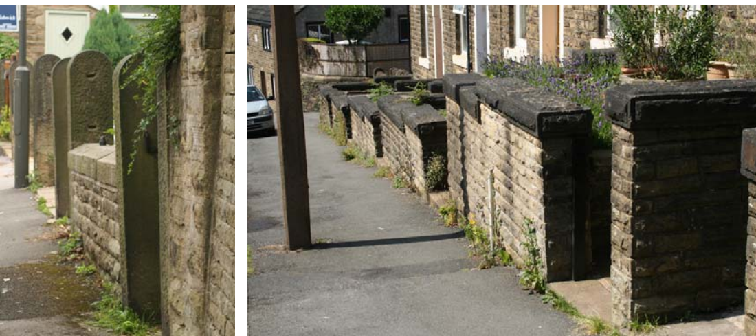
Stoops to gateways (left) and rock-faced even courses (right) shared by C19 cottages
