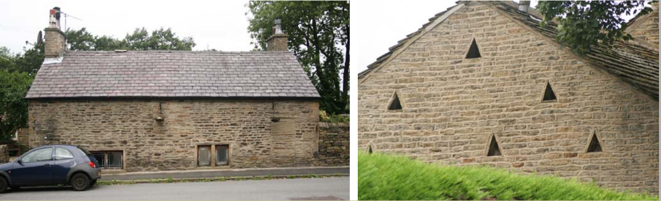
Former barn at 20 Hague Street (left) and ventilation slots at 8 Hague Street
