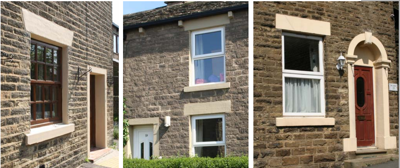
The evolution of the C19 cottage - from thinly-coursed gritstone with stone wedge lintels and narrow door lintels and jambs, to squared lintels, to doors with arched stone lintels and fanlights
