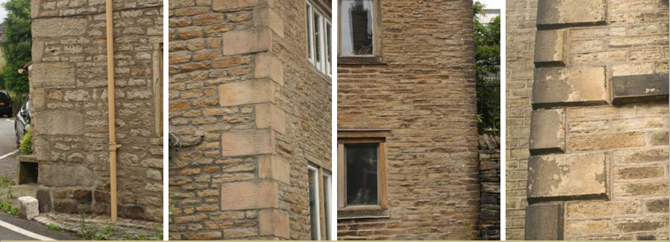
Narrow courses of walling stone with quoins or plain corners survive throughout the village
