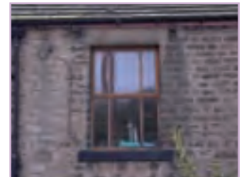
Windows should be set below the roofline and not break the continuity of the eaves. Dormer windows are not appropriate
