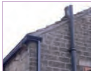
Downpipes and guttering should be discreet, black and located close to the eaves of the house
